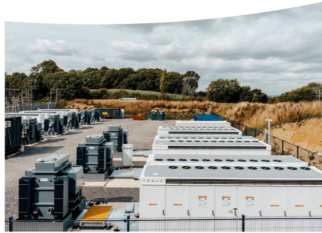
20 MW Hawkers Hill battery storage facility in Dorset.
