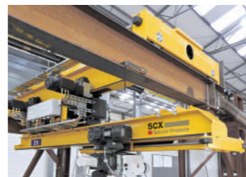
Sellafield PFSP cantilevered crane
