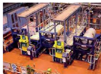
UF 6 Cylinder washing facility
