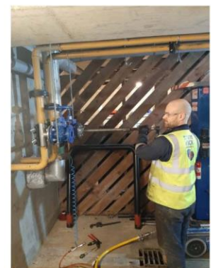
A new connection being made under live conditions using our under pressure system
