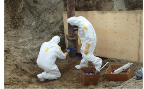
Canadian Nuclear Laboratories carrying out a pipe sealing operation on an active pipe using a bespoke FOAMBAG™ kit designed specifically for their project
