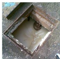
A foam filled chemical drain at Chapelcross
